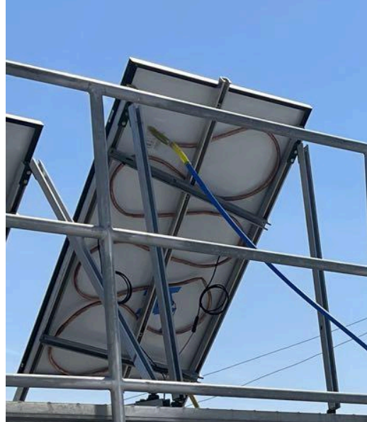
Figure 4. Bent copper tubing along the back of the PV panel.
